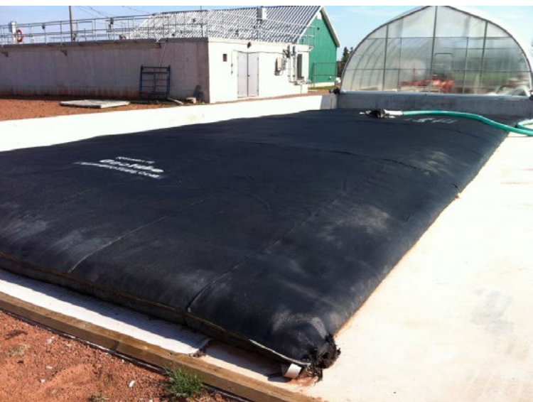
Biosolids are pumped at a rate of about 250 L/min into one of four Geotube containers that are positioned on a large concrete lay-down area.
