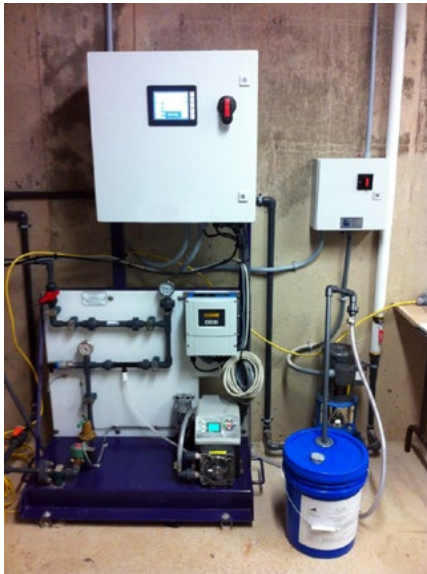
A VEPAS system monitors the flow rate and injects polymer directly into the biosolids line.
