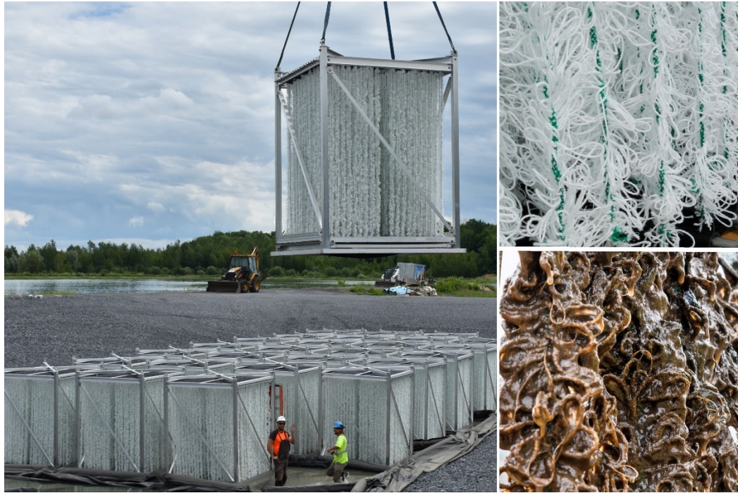
Figure 1. A BioCord system shown during installation into a municipal lagoon. A closeup of the clean BioCord media (top right) and a the media after establishment of a robust biofilm (bottom right).
