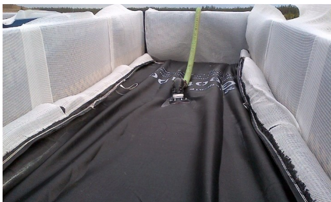
Figure 10. Two Geotube containers are set up in roll-off bins to collect and dewater the arsenic sludge. Once full, operators can easily move the bin to an onsite storage area, tip out the Geotube, and replace it with a new one.
