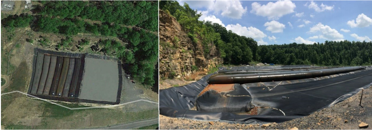
Figure 5. At left, an aerial view of the dewatering cell at the Omega Mine At right the third layer of Geotube containers shown in 2018.
