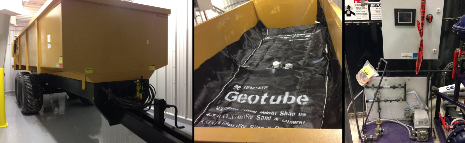
The hydraulic dump trailer shown with a newly installed Geotube® container. The VEPAS (right) mixes and activates polymer in a single step, then injects it directly into the sludge feed line.
