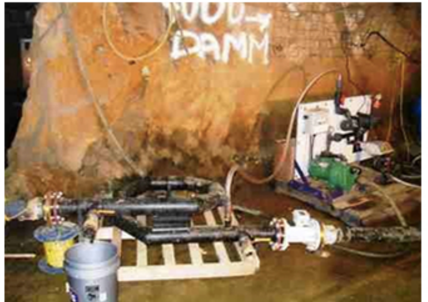
Bishop Water Vepas 100 Chemical Injection Unit and custom fabricated mixing chamber in Northern Ontario
