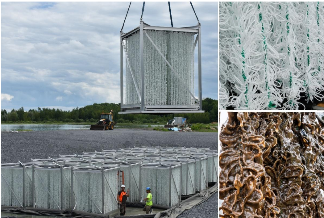
FIGURE 1. BIOCORD REACTORS ARE SHOWN BEING INSTALLED INTO A LAGOON CELL (LEFT) TO IMPROVE TREATMENT CAPACITY AND PERFORMANCE. THE ROPE-TYPE MEDIA (UPPER RIGHT) SUPPORTS THE GROWTH OF A ROBUST, COLD-TOLERANT BIOFILM (LOWER RIGHT) THAT INCREASES REMOVAL OF AMMONIA AND ORGANICS.
