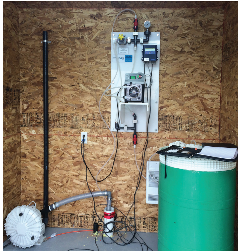
pH adjustment system and blower
