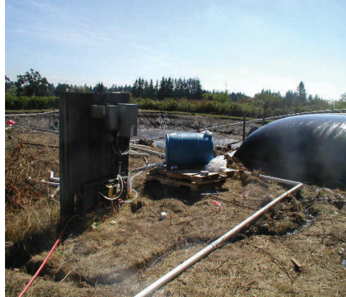
Figure 2. Polymer metering system with Geotube® unit.
