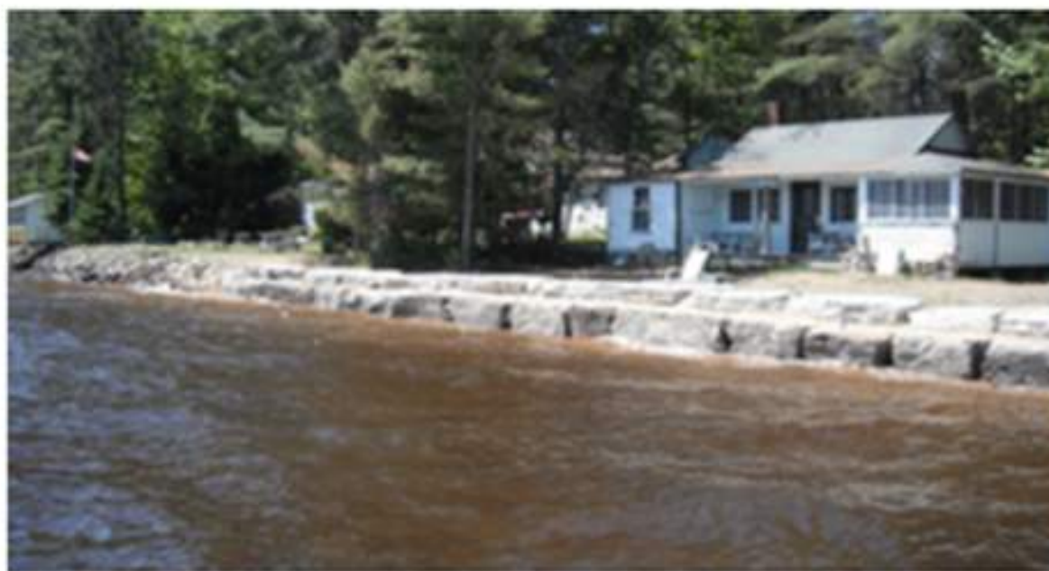
Shoreline in June 2014 . No movement was visible in the Geotube or the Armour stone that covers it.
